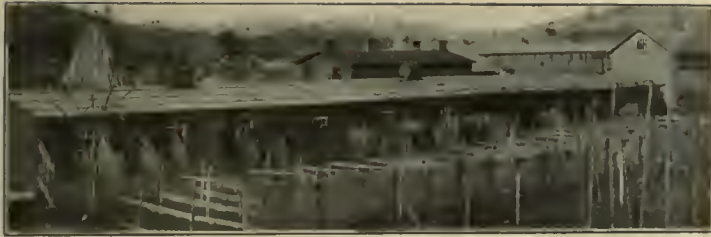
Brooder house, roof covered with PAROID, White Leghorn Poultry Yards, Waterville, N. Y.
