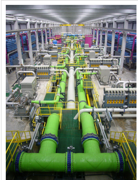
Reverse osmosis desalination plant in Barcelona, Spain
