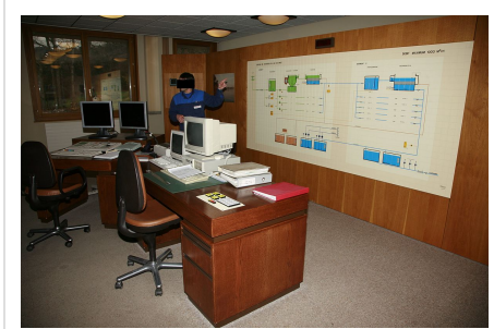
Control room and schematics of the water purification plant to Lac de Bret, Switzerland
