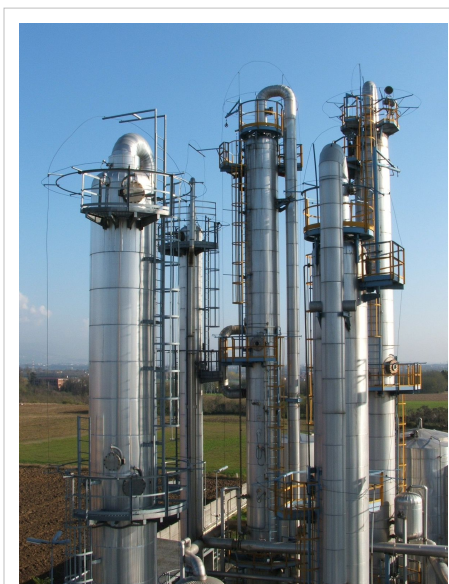
Typical industrial distillation towers
